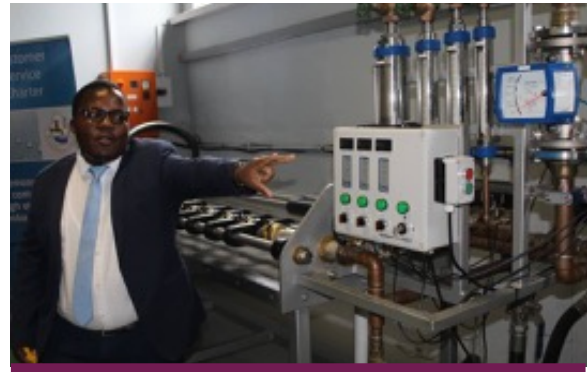
Eswatini Water Services Corporation (EWSC) – Mechanical Meter Verification Laboratory transitioned on time
